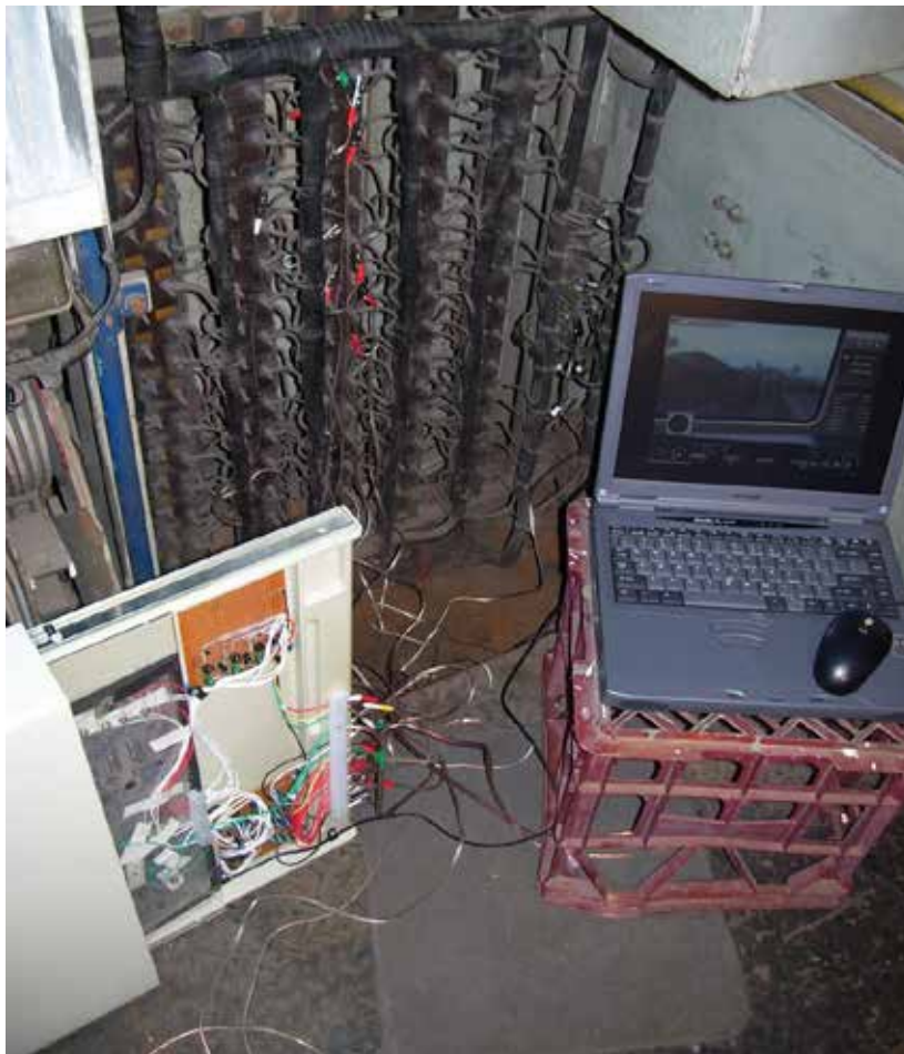
Interface Unit and Computer in the No. 2 End H.T. Compartment Note temporary wiring and use of alligator clips. (Photos: Steve Corrigan)
