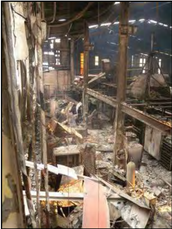
Above: The burnt out remains of what was once the Workshop and Office within the Bottom Points depot. Out of all this despair there is hope and some good news to share.
