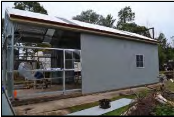
Above: Frame completed cladding is applied to the roof and walls. Photo: Andrew Tester
