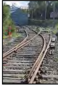
Left & Below: The No 2. Ash Siding complete except for tamping. A new set of points has been partially installed for a new bogie siding will branch off to the left as you look towards the shed. Photos: Andrew Tester
