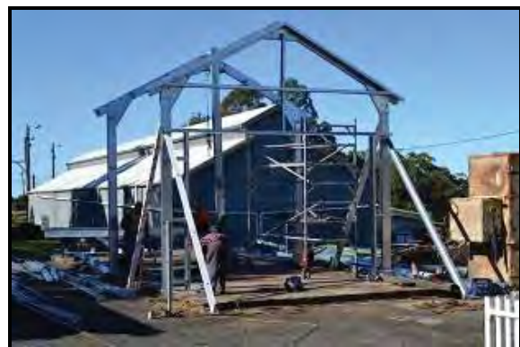
Above: The first sections of framework are assembled – 1 July 2013 Photo: Ted Mullett.
