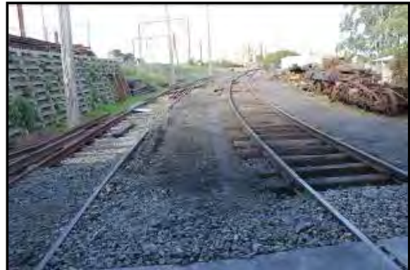
This short section of track is where the tram departs from and during the 1980s a slab of concrete was poured over this section by depot staff, burying the rails and timbers until recently.
