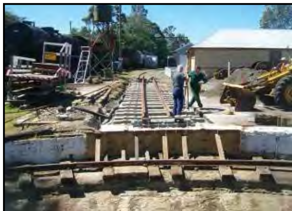
Below: Replacement sleepers and rail sit atop the new bed waiting to be fixed in place. Photo: Andrew Tester.
